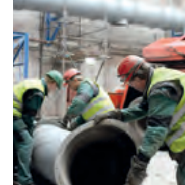
Dedusting of the Steel Plant
