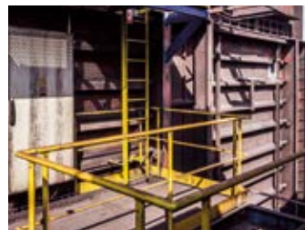
Increasing efficiency of de-dusting the material routes, Sinter Plant, northern part
