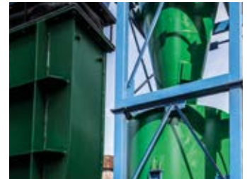
De-dusting of system of charging containers of ore bridge
