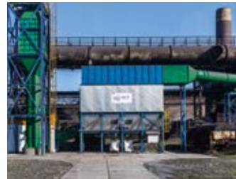
De-dusting of cleaning station for torpedo cars
