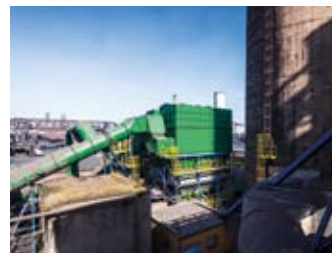
Blast Furnace 2 - charging system de-dusting
